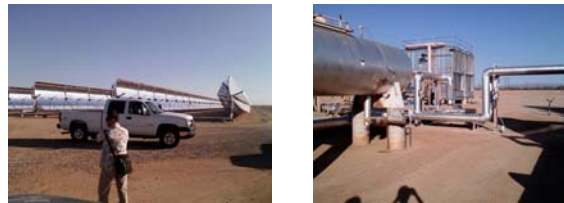
(a) Parabolic trough solar receiver (b) heat exchanger and cooling tower
